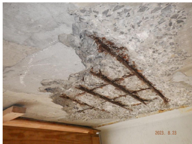
TYPICAL DECK DETERIORATION PHOTOS
